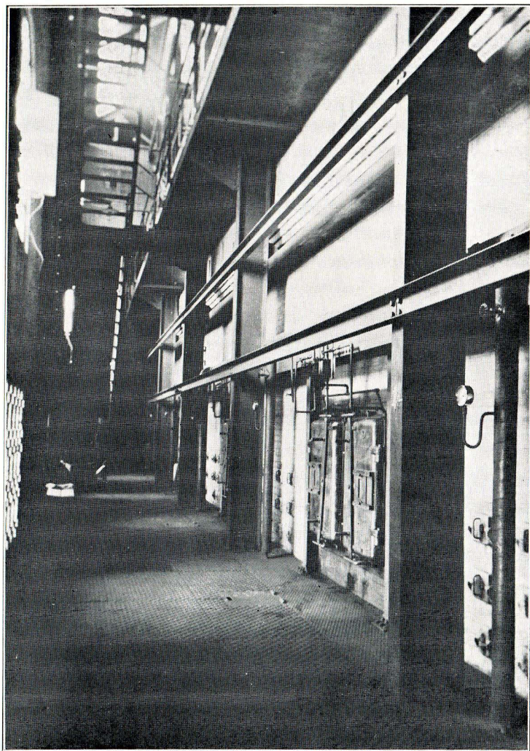
W-D KONTINUERLIG VERTIKALOVN - GENERATORER W-D CONTINUOUS VERTICAL RETORT OVEN - PRODUCERS
